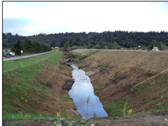
Photo 21. Newly restored section of the main Johnson Creek reach, looking upstream of the inlet to the outfall to the Green River (fish passage ID 50000, partial barrier). The culvert and flood gate were replaced with a fish-passable structure (passable under most flow conditions) under the mitigation for the adjacent Tukwila South project. (Date: Fall 2011)
