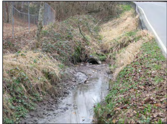
Photo 8. Southgate Creek: view of inlet to City-owned culvert under S 132nd Street (fish passage ID 50015, partial barrier). There was no flow through the culvert due to sediment blockage at the time this photo was taken. (Date: 2/3/2011)
