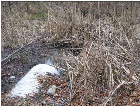
Photo 9. Southgate Creek: view of pipe outlet into the wetland that conveys the main branch (fish passage ID 50015, partial barrier) just upstream of SR 599. (Date: 2/3/2011)
