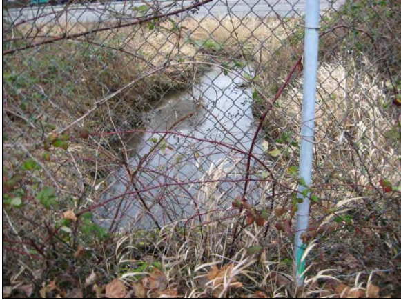
Photo 1. East Fork Riverton Creek: view downstream from the outlet of the 2,000-foot long pipe along East Marginal Way S (fish passage ID 50005, partial barrier). (Date: 2/4/2011)
