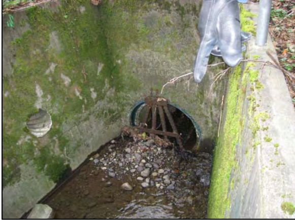
Photo 11. West Fork Southgate Creek: view of the inlet to the long culvert under S 133rd Street (fish passage ID 50021, total barrier). The steep gradient as well as the structures shown here and in Photo 12 combine to act as a total fish passage barrier. (Date: 2/3/2011)
