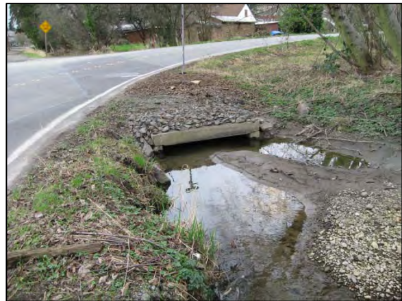
Photo 10. East Fork Southgate Creek: view of the east end of the culvert under 44th Place S (fish passage ID 50016, non-barrier). Flow from the west fork was diverting into a pipe at S 133rd Street, instead of passing into the main channel, due to channel gradient and sediment blockage. (Date: 2/3/2011)
