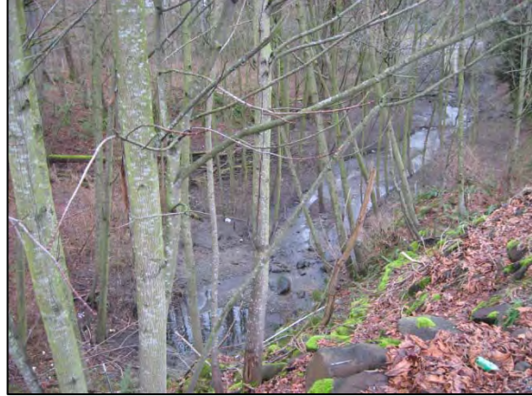
Photo 19. Upper Gilliam Creek: view downstream from outlet of the culvert underneath Southcenter Boulevard (fish passage ID 44989, total barrier). In addition to the culvert identified by WDFW as a total barrier, the flow appeared too low for adult fish through this length. (Date: 2/4/11)
