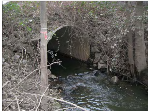
Photo 14. Gilliam Creek: view of the outlet of the WSDOT-owned culvert under the south shoulder of I-405 (fish passage ID 40864, partial barrier). This 1,100-foot long culvert is identified as a partial fish passage barrier likely because of high discharge during high stream flows due to its length. (Date: 2/3/2011)
