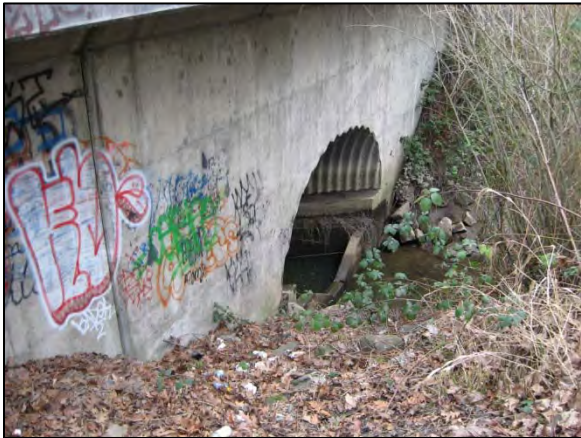
Photo 7. Southgate Creek: view of the outlet of the culvert under Interurban Avenue S (fish passage ID 50013, partial barrier). The fish ladder just inside the culvert is considered a partial fish passage barrier because low flows did not appear sufficient to allow fish to jump over the weirs. (Date: 2/3/2011)
