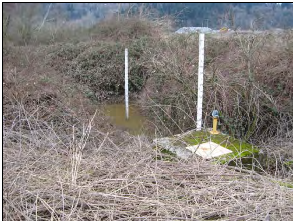
Photo 20. Johnson Creek: view upstream of the old inlet to the outfall to the Green River (fish passage ID 50000, partial barrier). The flap gate and outfall were replaced with a fish-passable structure (see Photo 21). (Date: 2/3/2011)
