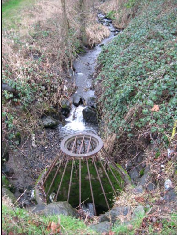
Photo 18. Upper Gilliam Creek: view of the Gilliam Creek RDF structure (fish passage ID 45078, partial barrier). This feature was identified as a partial barrier by WDFW, but appeared to be a total barrier during the windshield survey. (Date: 2/4/11)
